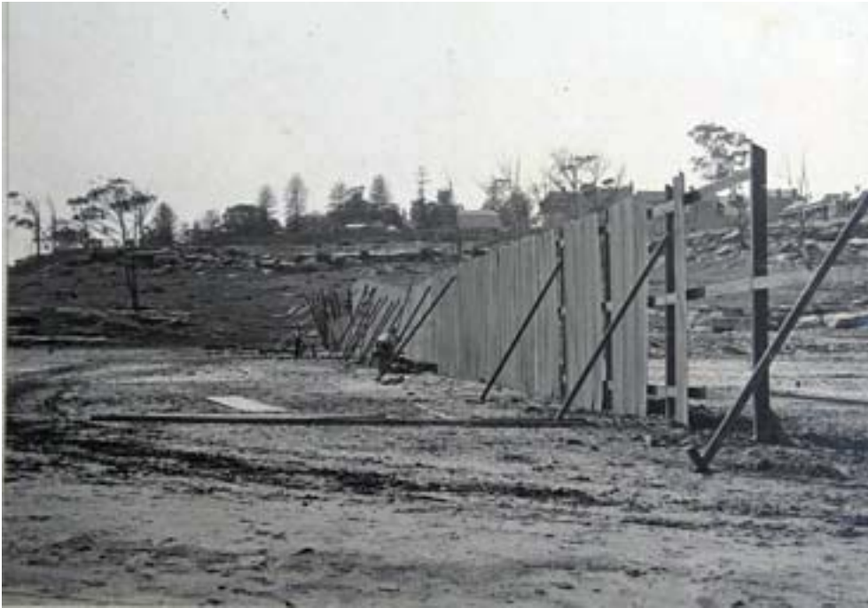
Figure 3.3: Construction of the paceway boundary fence 1909. Image no 3863 from Allen family album
