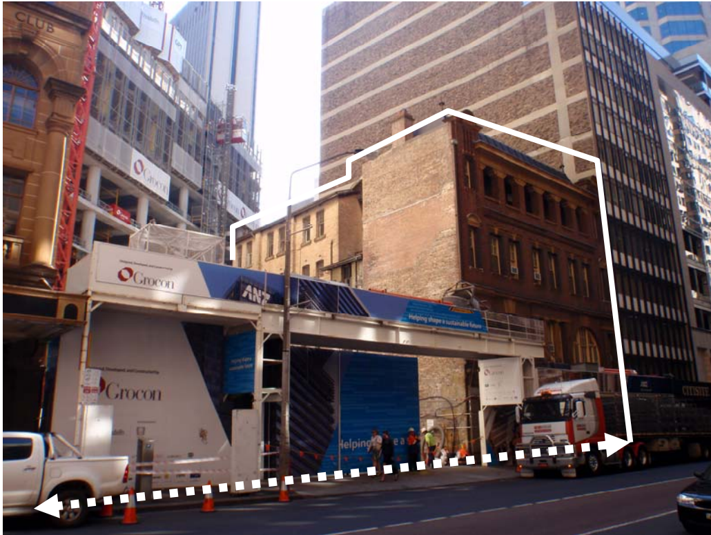
Figure 2: Castlereagh Street frontage with Legion House highlighted with Citisite House in the background
