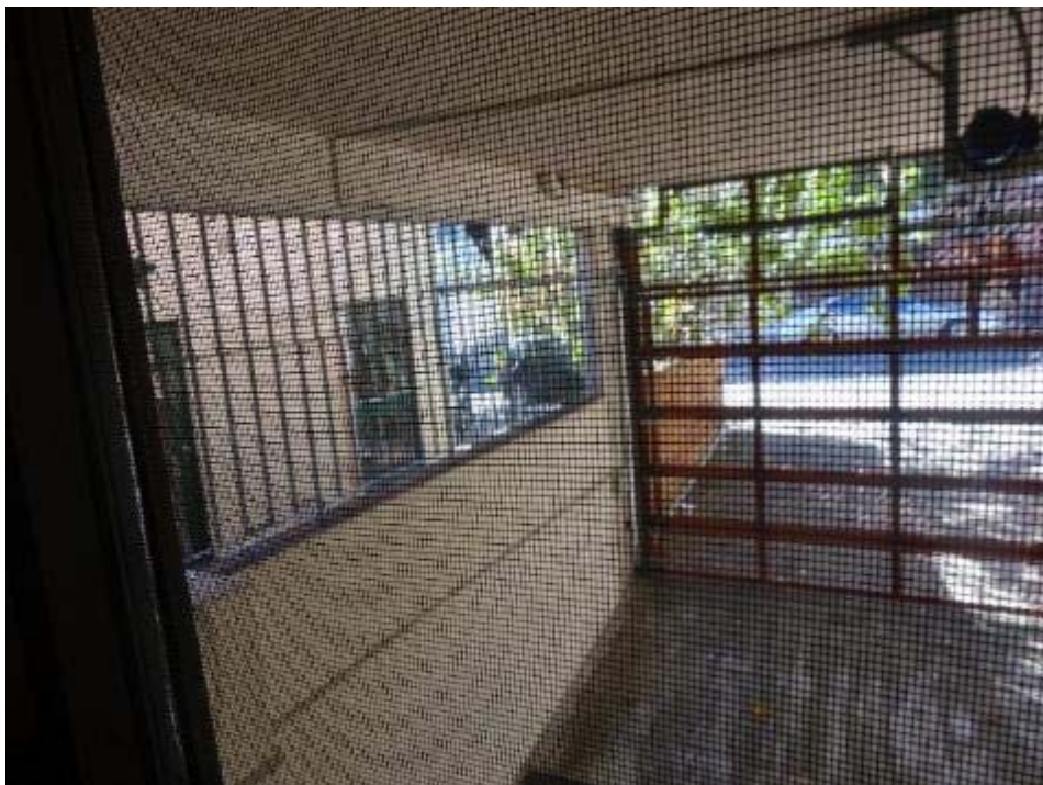
Figure 2: Internal view from bedroom over driveway and existing opening to the adjoining subject site
