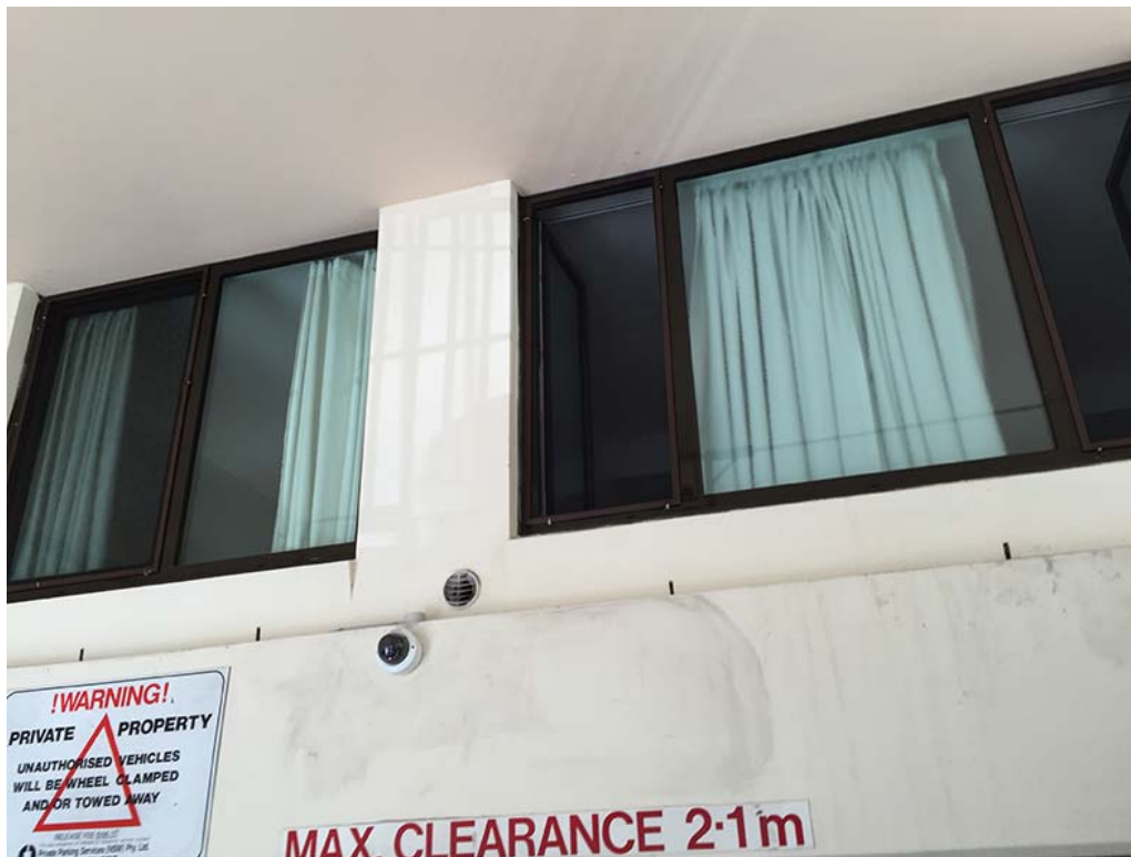
Figure 5: Windows in question from driveway
