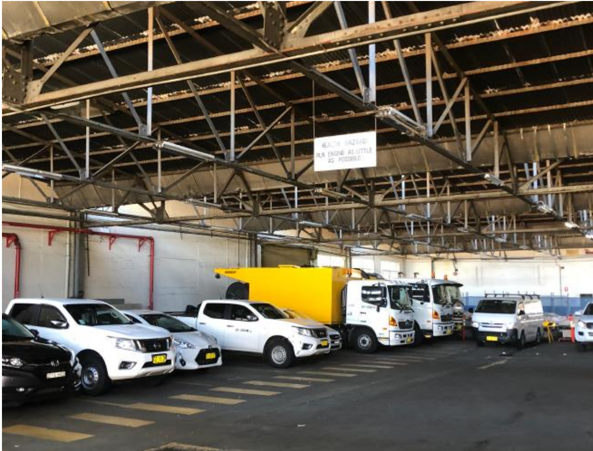
Figure 4: The interior of the garages building with the rear of the Bay Street wall to the left
