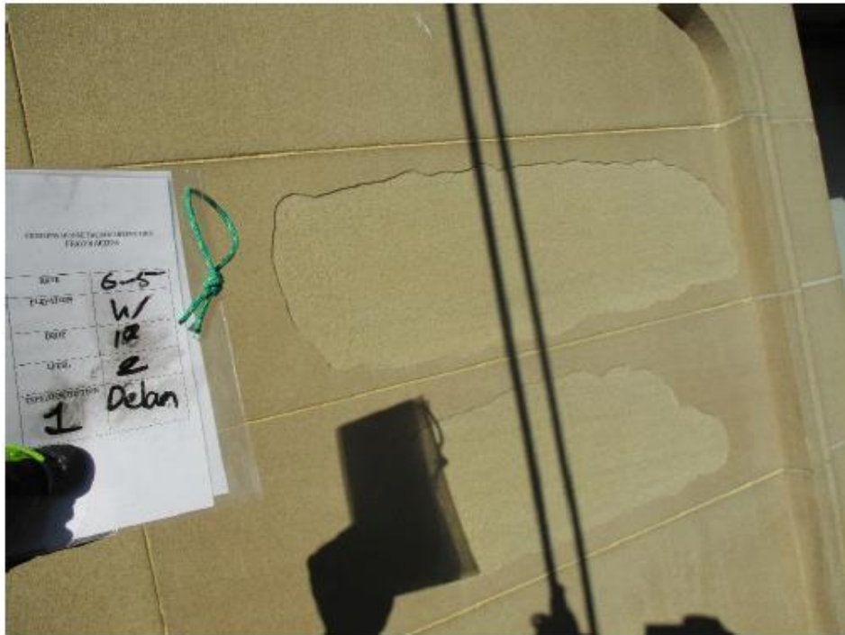
Level 2: weathering of sandstone wall
