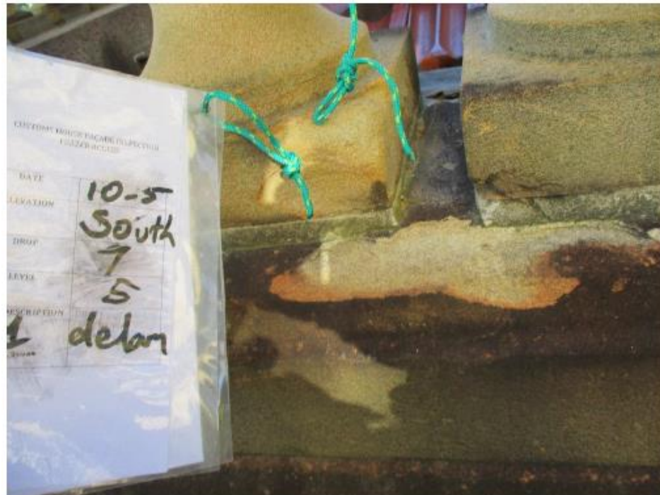
Level 5: sandstone deterioration at base of balustrades
