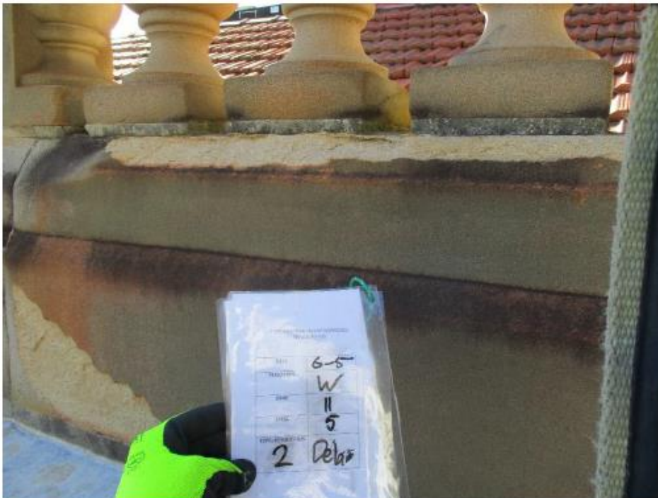
Level 5: deterioration at base of sandstone balustrades
