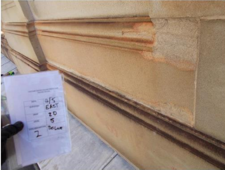
Level 5: deterioration of sandstone wall
