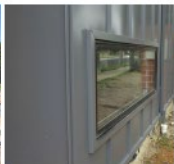
MDC1 MDR1 METAL DECK CLADDING / ROOFING STANDING SEAM ZINC CLADDING Blue Grey Zinc
