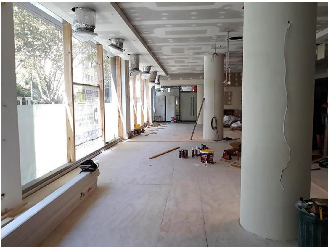
Figure 5: Internal fit-out works currently being carried out as approved by CDC no. NW18/3279.
