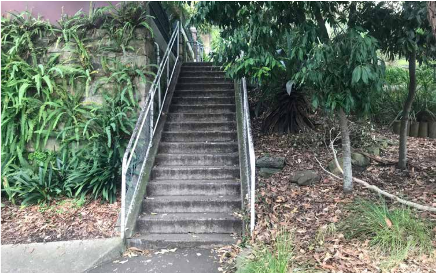
Image 2 - Photo of access stairs to Palmerston Avenue from Glebe Light Rail Station
