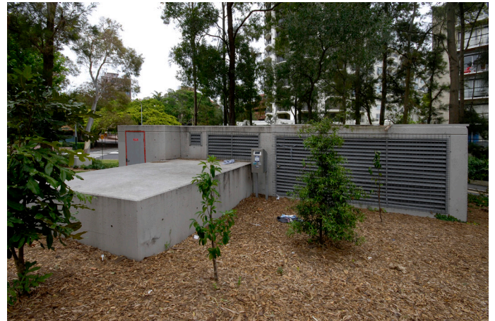
Existing carpark vents - visual barrier
