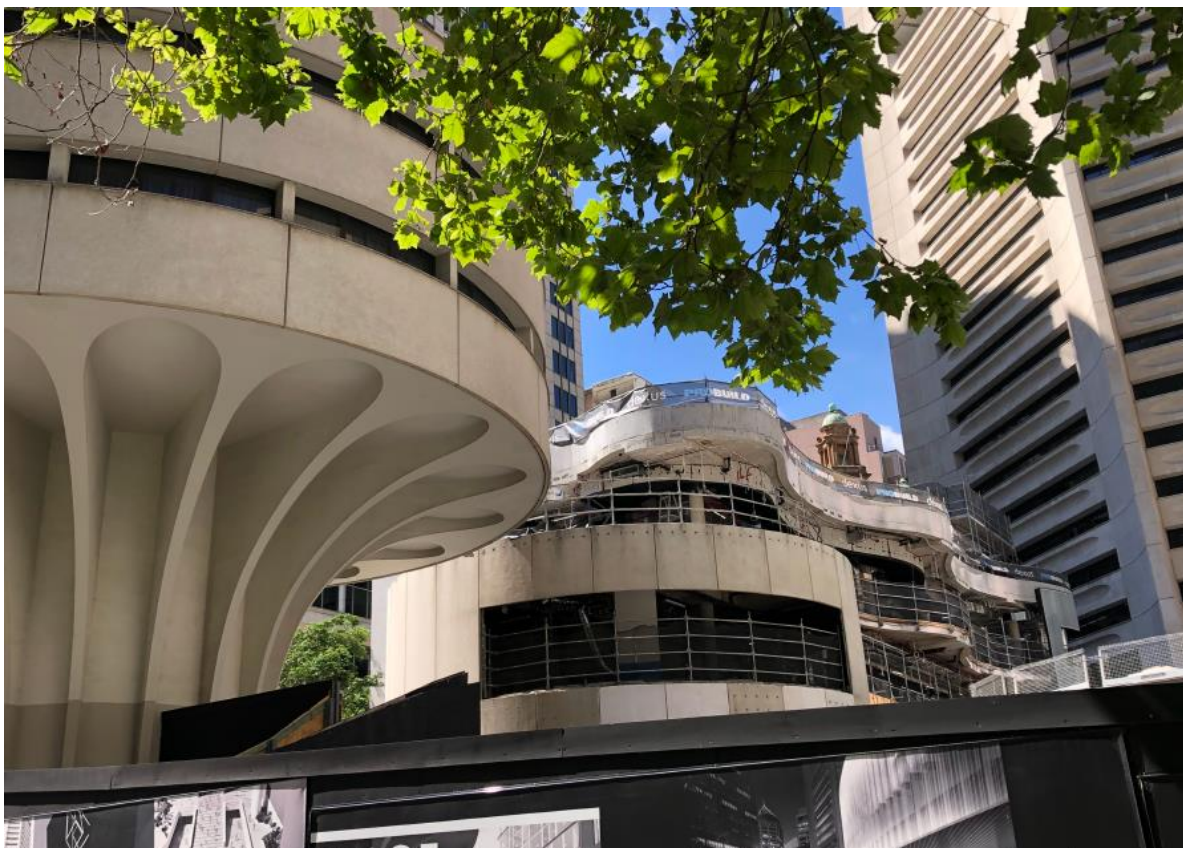
Figure 4: Site as viewed from Martin Place, with subject tenancies currently under construction
