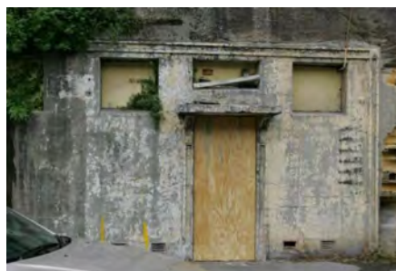
Condition 5 – Very Poor
