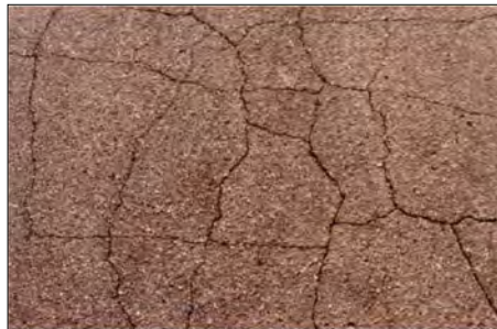
Condition 5 – Very Poor
